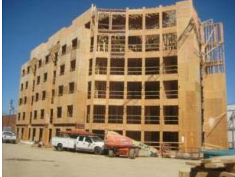
Big Switch: York Residential decided to go with wood-frame construction instead of concrete to make the five-story North Tract Lofts in Arlington, Va., financially feasible.
